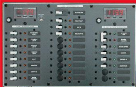
High quality AC/DC electrical panel is only one component of a well-engineered electrical system.
