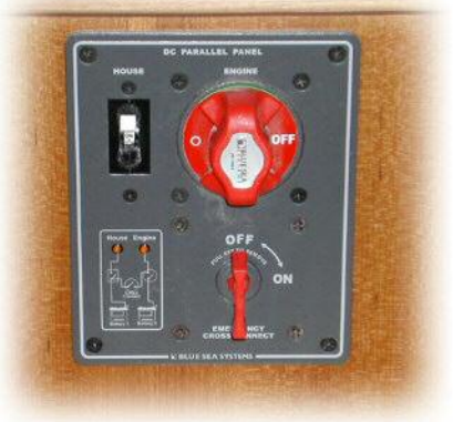
Battery cut-off switch for ultimate security and safety and emergency transfer switch if the need arises.
