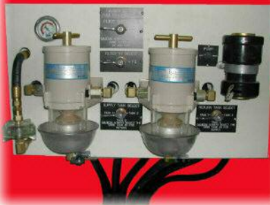
Dual fuel systems for safety are combined with dual huge capacity tanks.
